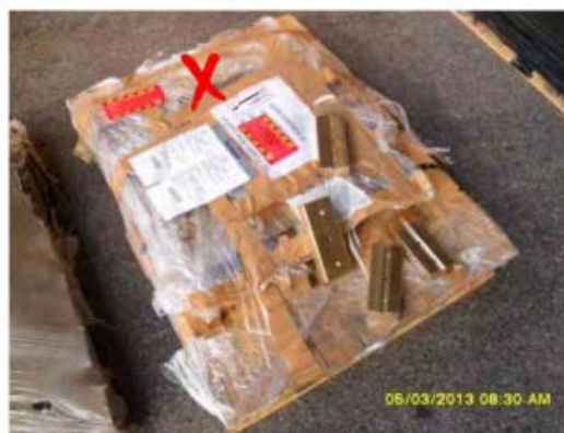
Shrink wrap was the only restraint applied to this load which proved inadequate prior to it being sent to site.
